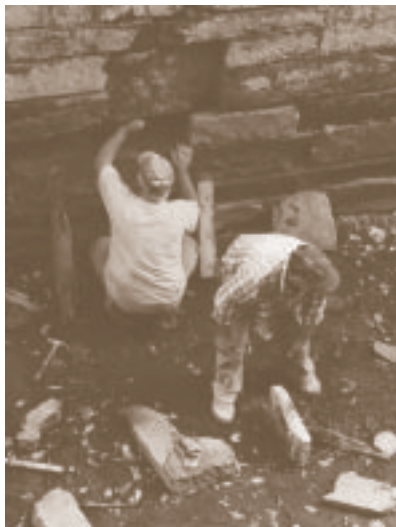
The Bi-State masons at work at the bottom of Locks 15/16 in Smithtown.
