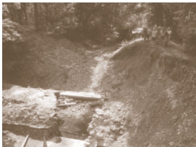
The collapsed High Falls Creek Culvert. Photo by Hal Pschunder.
