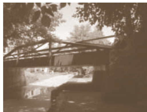
The new utility chase cover on Mechanic Street Bridge in downtown New Hope.
