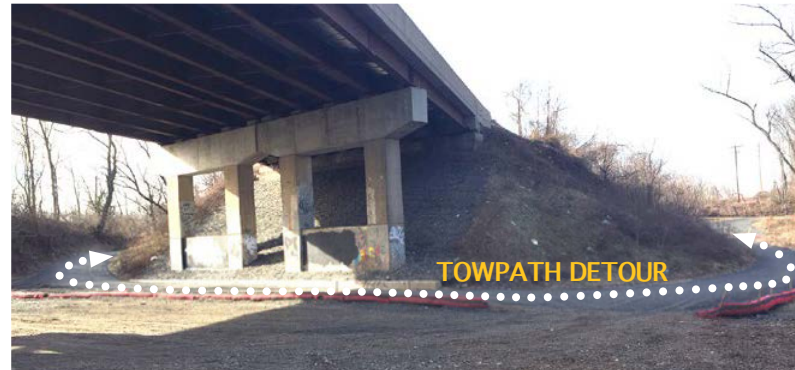
The new towpath trail detour circles the Tyburn Road piers, well away from the railroad tracks. The Canal runs through a culvert pipe to the north of the piers.
