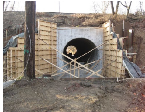
The Conrail embankment passageway with its wing wall formwork still in place.
