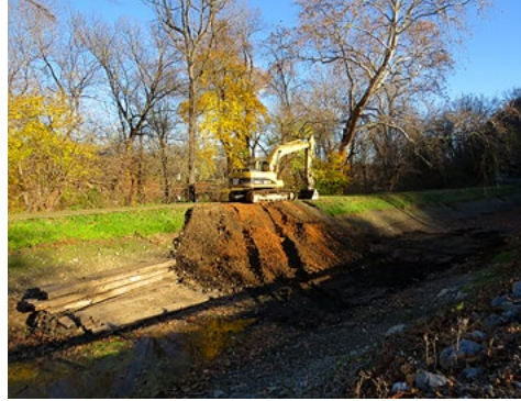
The area where a sinkhole had been repaired with "flowable fill" is covered with clay to restore the Canal's ability to hold water.
