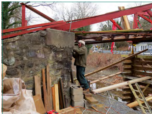
Contractor Randy Myer is determined to get the restoration of Woody's Camelback Bridge done this winter.
