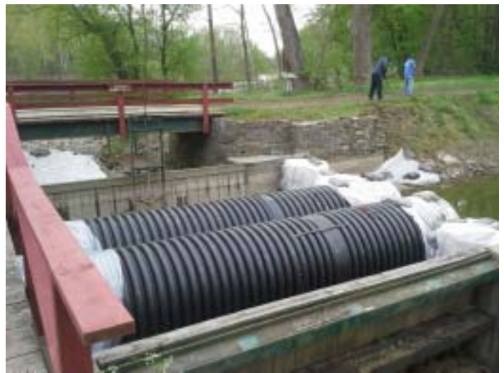
These pipes are allowing water to flow through the damaged Kleinhans Aqueduct.
