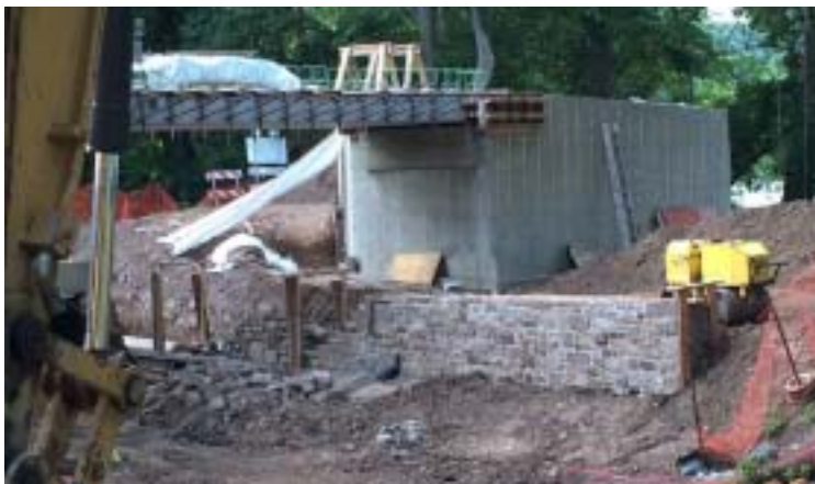
Work on all the component parts of the Redfield Bridge project is underway.
